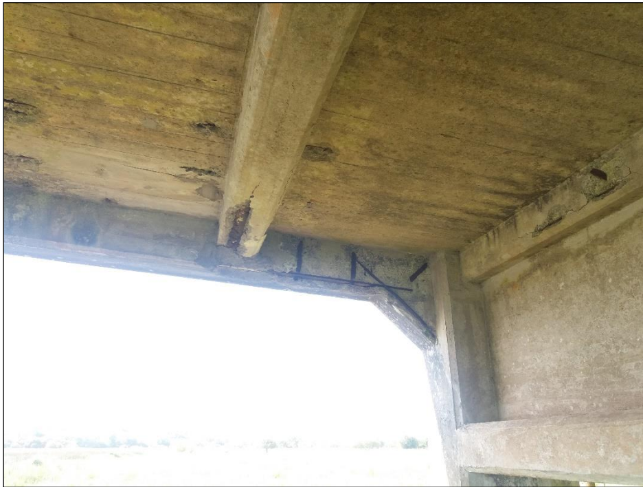
Figure 3 - Example of extensive spalling and reinforcement corrosion
