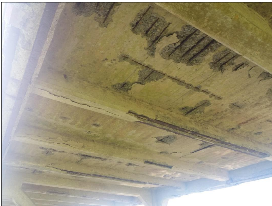
Figure 2 - Example of extensive spalling and reinforcement corrosion
