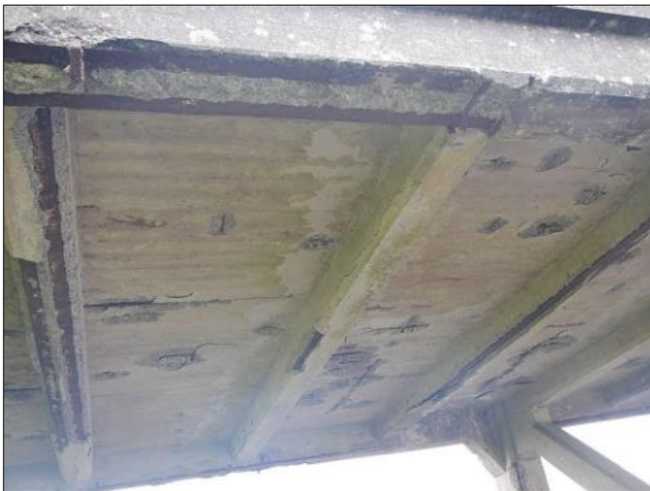
Figure 4 - Example of extensive spalling and reinforcement corrosion
