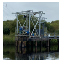
Regional water supply intake
