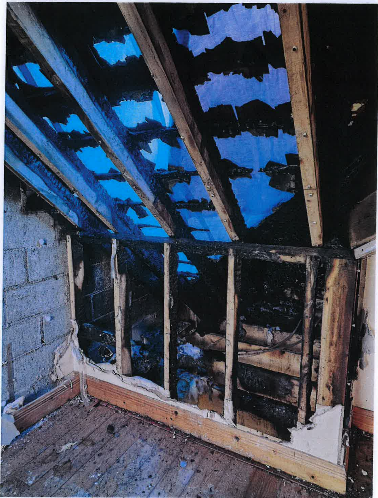
Photograph no. 8 Shows the attic area close to where the fire broke out. All this section of roof needs to be replaced.
