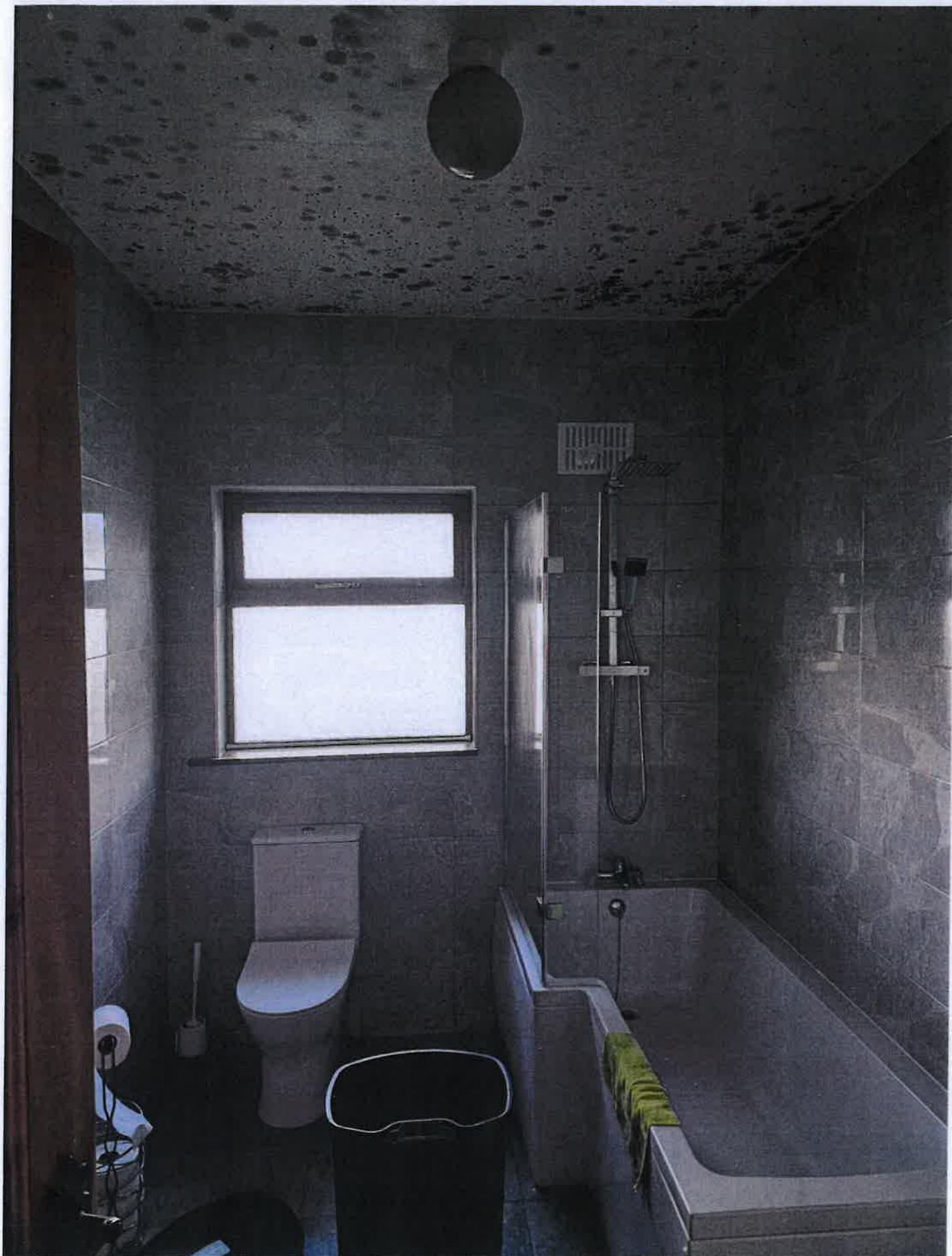
Photograph no. 7 Taken in the bathroom towards the rear of the dwelling. Note: the damage to the ceiling.
