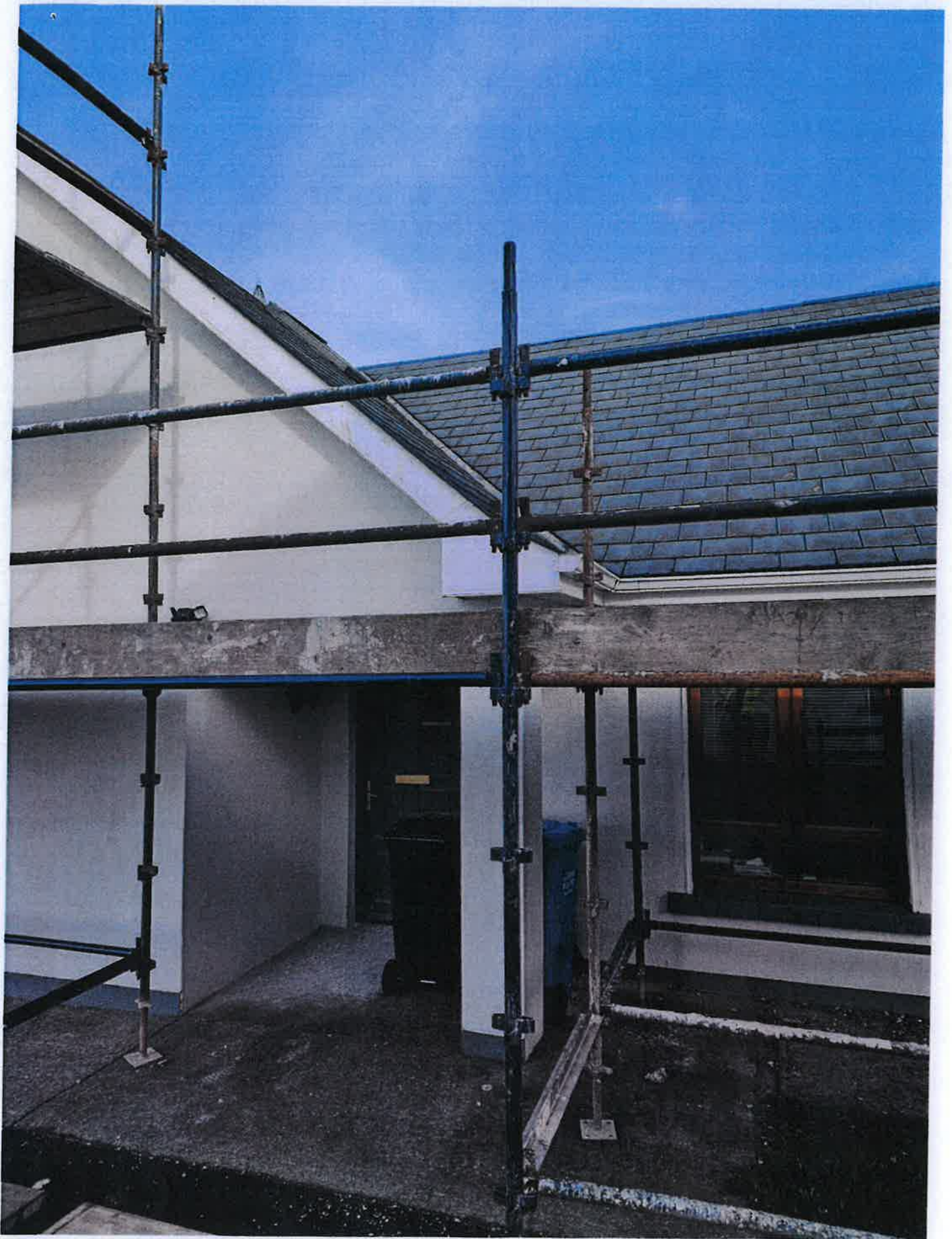
Photograph no. 2 Shows the roof area over the entrance door at the front of the dwelling which is not damaged.
