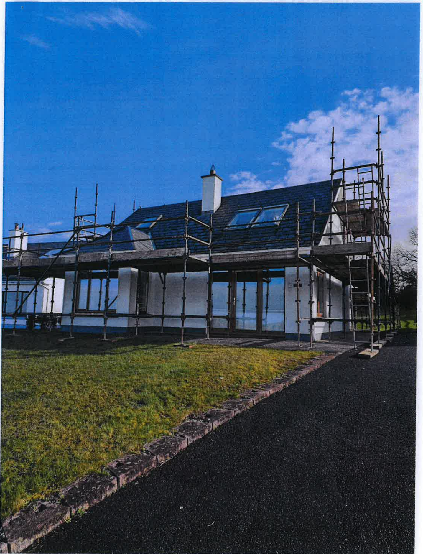
Photograph no. 3 Shows the side elevation to the left-hand side of the front door, which is also not damaged.
