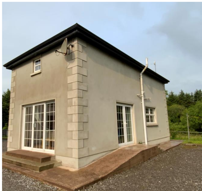
Fig.5 Structure on site varies from that permitted under P.06/689
