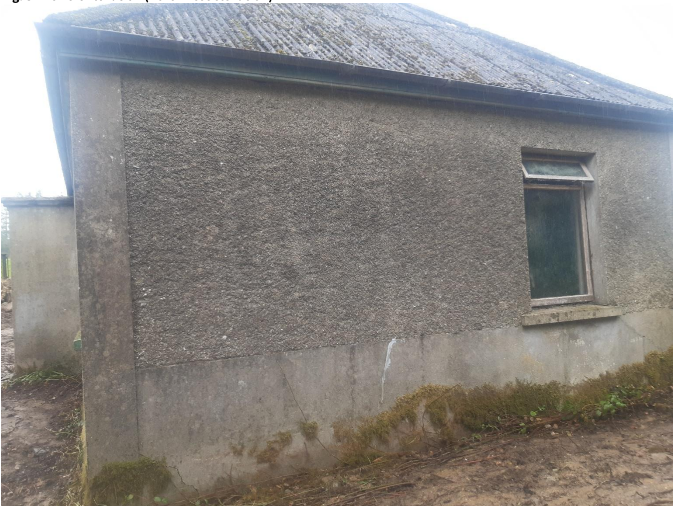
Fig. 4. The Right Elevation (southeast elevation)
